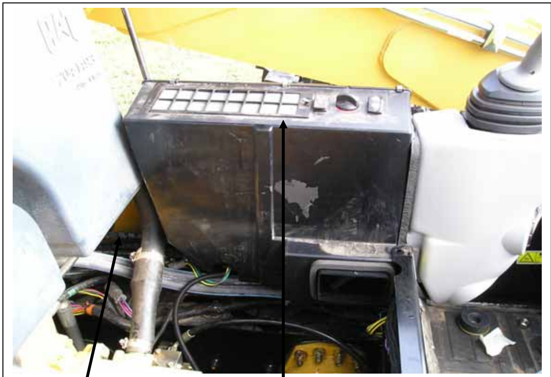
A/c lines and relay control wire.
