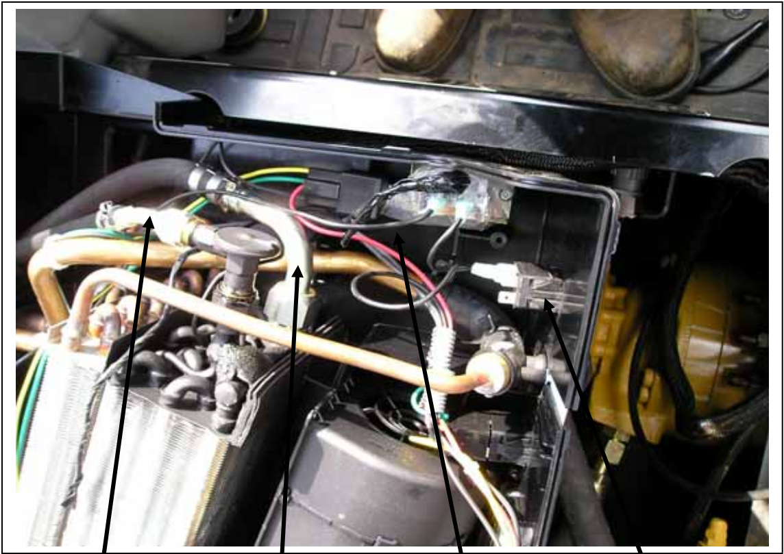
5/16" 45° fitting at expansion valve.
